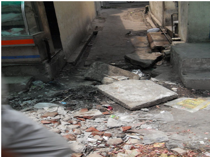
OPEN DRAIN, NO SEWERAGE
