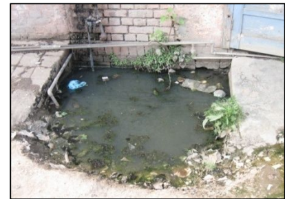
Fig no.87: View of Blocked Sewer at Mahan Singh Gate
